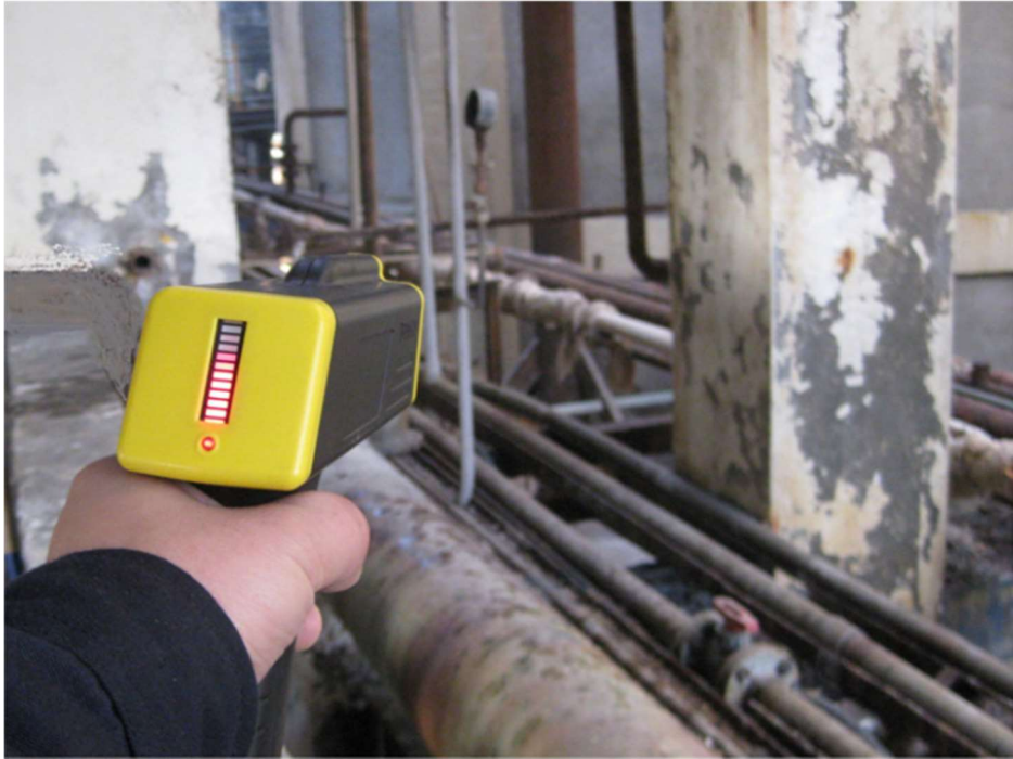
Fig. 25 Photo of the directivity-based ultrasonic leak detector (DULD)
