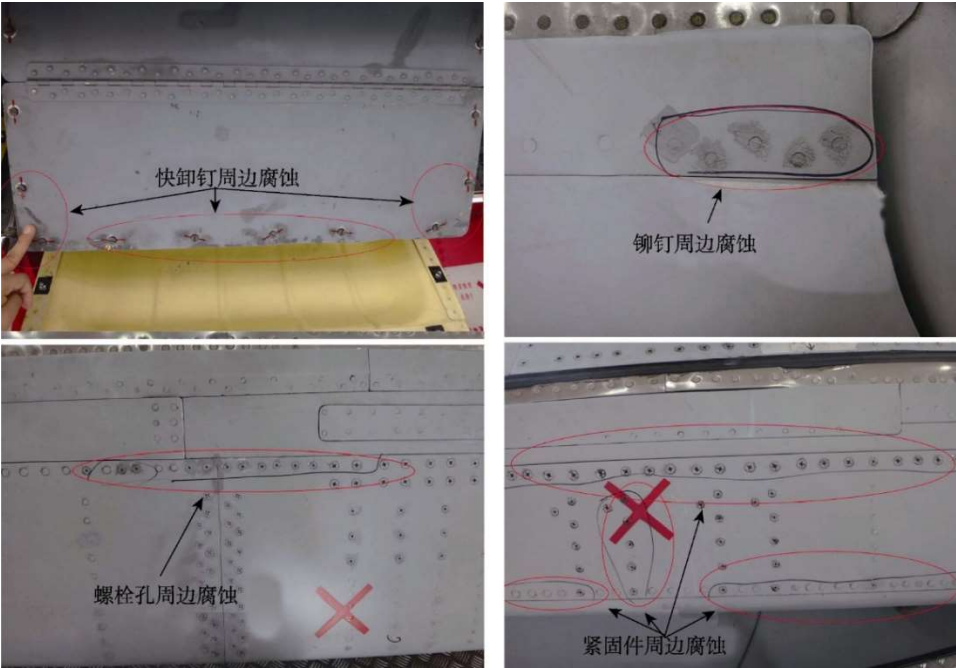
Fig. 3 Corrosion around fastener holes [14]
